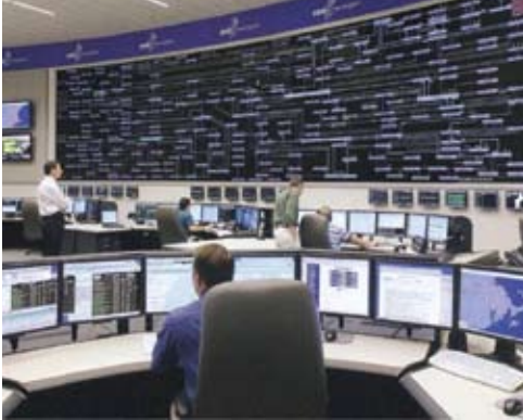
Control room of a transmission system operator
